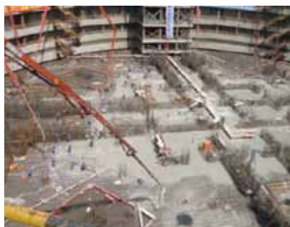
Fig 5.: Aerial view of the raft foundation placement of a major high rise in China
