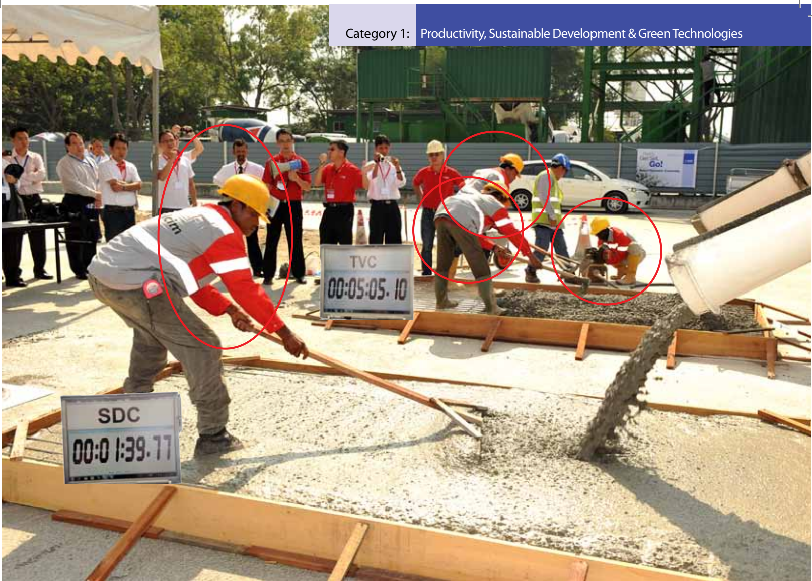
Fig 4: Field demonstration of the savings in labour and in time for placement of conventional vibratable concrete vs. low fines self consolidating concrete (Smart Dynamic Concrete)
